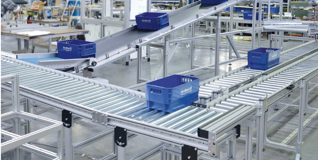
Interlink with RBM-P 2255 driven roller conveyors and RBS-P 2066 gravity roller conveyors for mail crates
