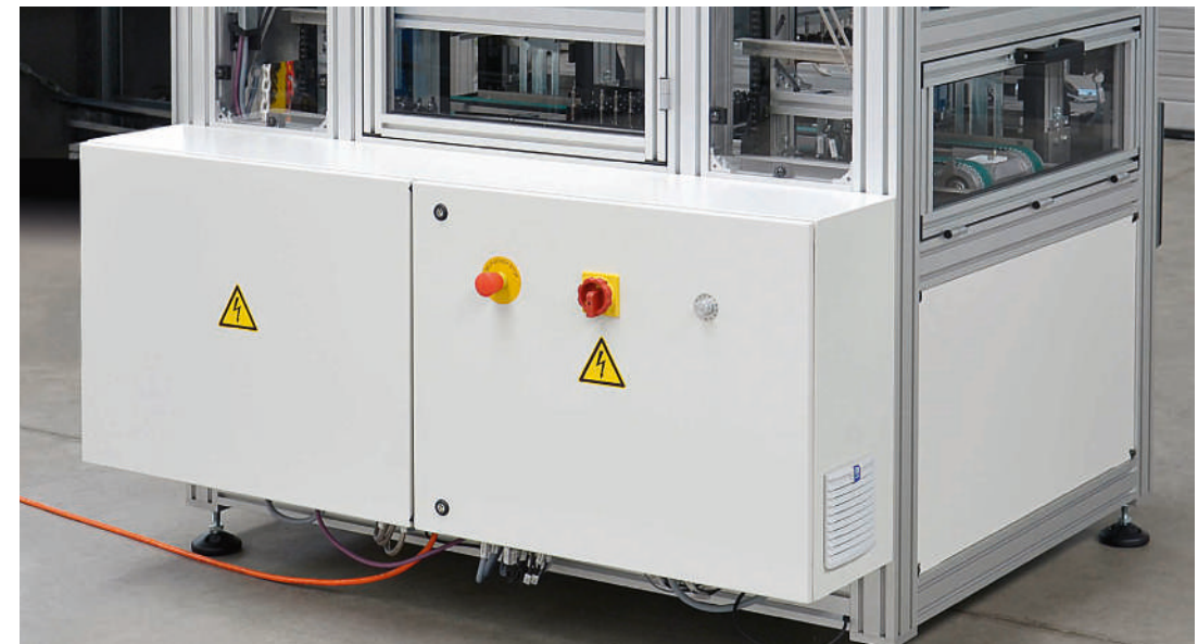
Control cabinet attached on the frame and protective device combination
